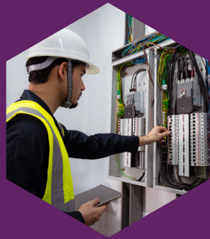
Electrical, Heating and Ventilation Contractors
